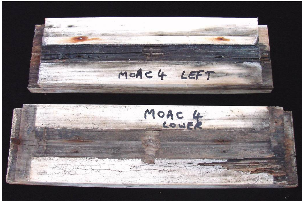
Figure 9. TBTN LOSP-treated E. regnans window MOAC4, painted. Lower piece shows upper face of bottom sill with 35+ mm brown rot in the left end (reversed in photo) that was dipped after machining. Top piece shows inside face of left piece with 2 mm decay under beading (it also has 35+ mm decay at either end).
